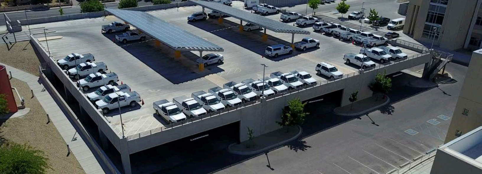
There are solar panels installed in many City facilities, including the parking structure at City Hall (above).
